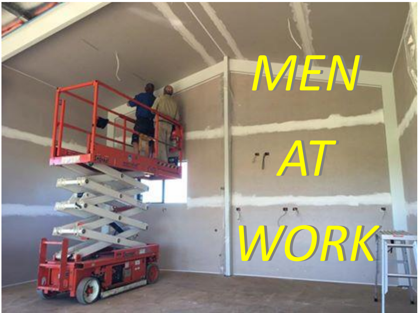
Jack and Ian working on the inside finish of the AAC storage shed
